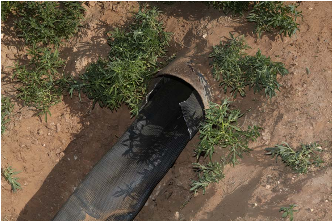
Photo showing a steel pipe culvert in which a hose is threaded through.
